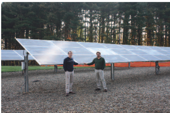
David Connors, left, Director of Supply Operations, and Michael Liberante, Treatment Manager, examine some of the new solar panels at Aquarion Water Company's Trap Falls treatment plant in Shelton.
